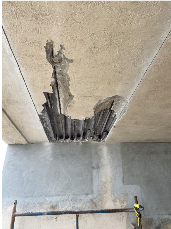
Picture 2: Ceiling repair in garage below unit 103
